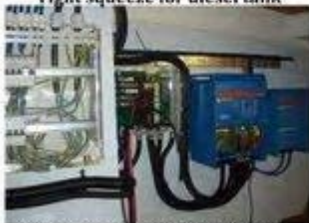
Complex electrical equipment
